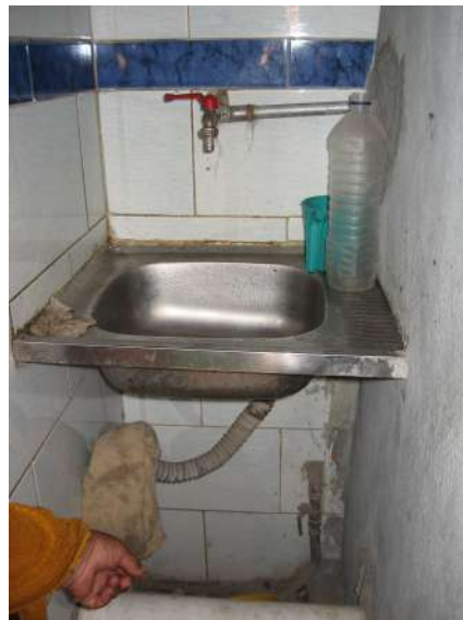
Hosh resident showing off a newly added w.c. and kitchenette sink. Water connections were installed easily due to proximity to the edge of the cemetery along Sook al-Hamam.
